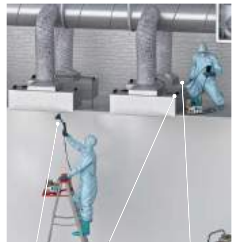
Leak testing with a photometer or DPC Injection of the aerosol from the plenum Upstream measurement of aerosol if no access from the room side from injection at the AHU
